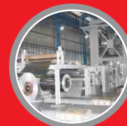
Aluminum Extrusion Plant
