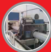
PVC Pipe Extruder Plant
